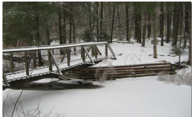
Bridges such as the above on Cole Hill State Forest in Albany County require maintenance in order to provide access for hikers, cross country skiers and other recreational users
