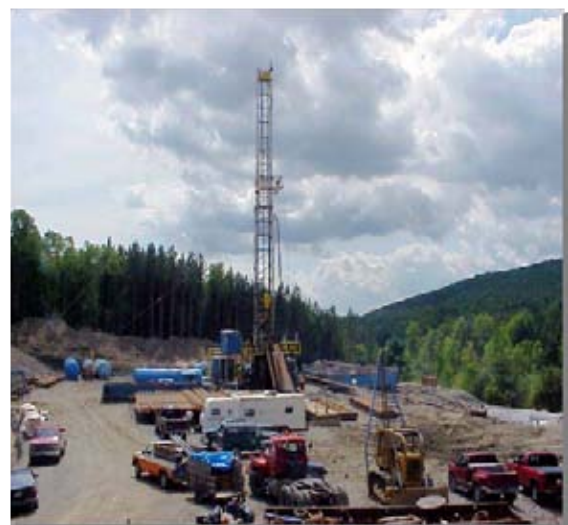
Well drilling on State Forest land over the Trenton-Black River natural gas formation
