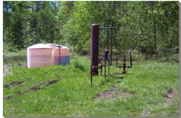
Natural gas production equipment on Hill Higher State Forest in Chautauqua County
